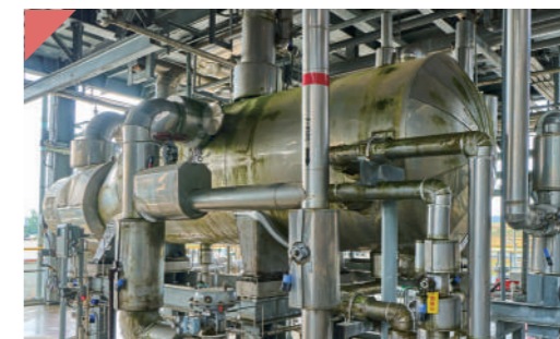
5 Dew Point Control Unit Cools and adjusts the dew point of natural gas for safe pipeline transport, preventing liquid buildup inside the pipeline.
