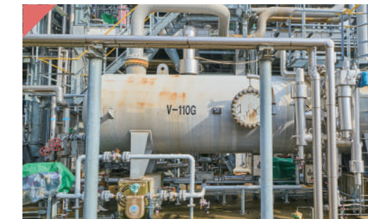
3 High-Pressure Separator Separates fluids into natural gas, oil, and water.
