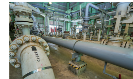
6 Delivery Manifold Room Delivers refined and processed natural gas through pipelines to city gas providers and other end users.
