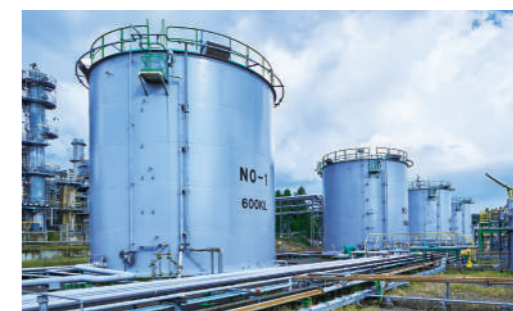
8 Condensate Tank Stores oil produced at the plant in tanks.
