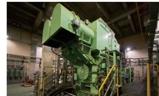
2 Low-Pressure Production Facilities Maintains maximum production even as gas field pressure declines.
